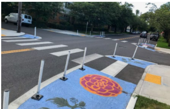
Intersection safety can be enhanced with painted bulb-outs and plastic bollards to shorten the crossing distance and slow motor vehicles, serving as a short-term "test" before making these permanent. Photo credit: Streetsblog
